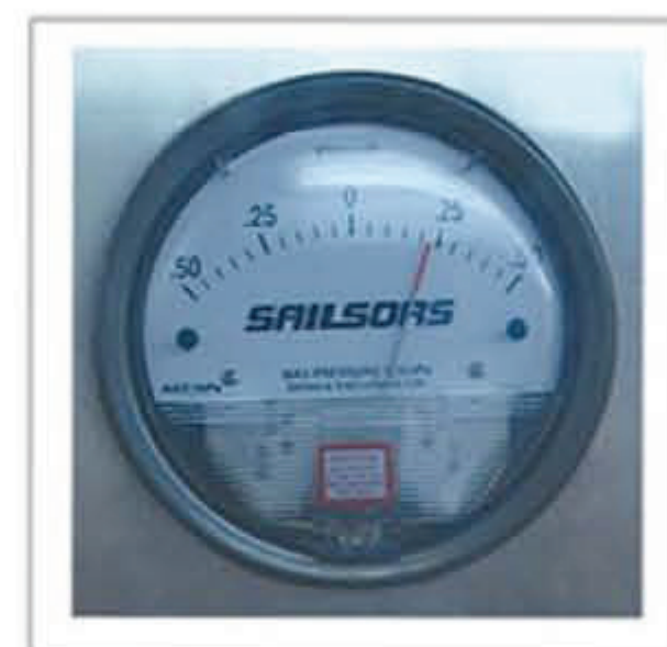
Pressure Meter Display the pressure of work zone.
